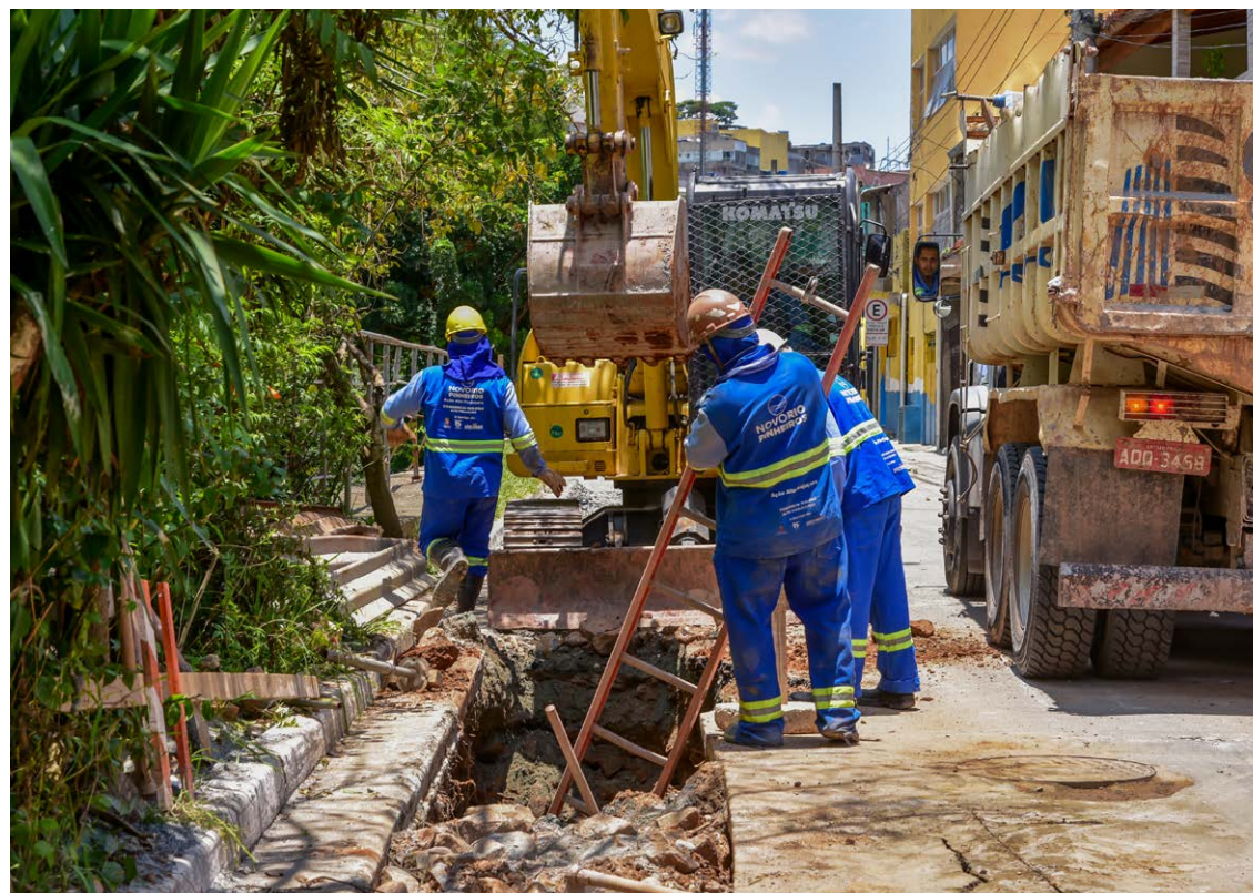
New Pinheiros River Program workers install collecting networks in the Alto Pirajuçara basin, in São Paulo
